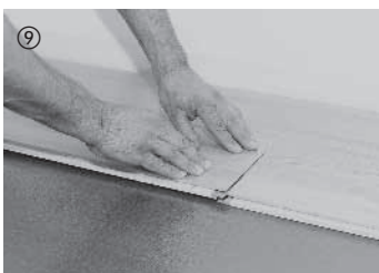
The board is then lowered in on the short side. Ensure here that the board is flush at the short side with the previously laid board. Pressure applied briefly to the side joint clicks in the board.
