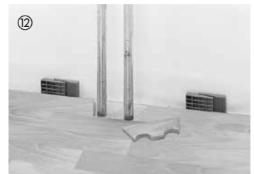
If radiator pipes protrude from the floor, drill or saw a cutout into the board (the size of the cutout depends on the radiator pipe and the required expansion space).
