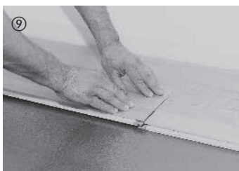
⑨ The board is then lowered in on the short side. Ensure here that the board is flush at the short side with the previously laid board. Pressure applied briefly to the side joint clicks in the board.
