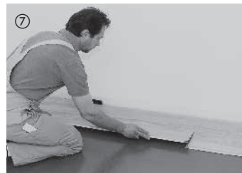
⑦ The next row is started with the leftover piece of the first row (short side offset of at least 50 cm). This considerably reduces waste. The rest of the installation is performed board-by-board. First, the boards are angled into the previous row along the long side by applying a small amount of force.
