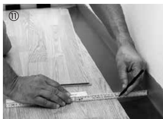
⑪ Cut to size and fit in the boards of the last row. Leave a gap of 10 to 15 mm between the boards and wall.
