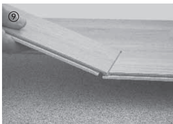
⑨ Insert the end of the next board of this row into the mating end of the board you just installed.
