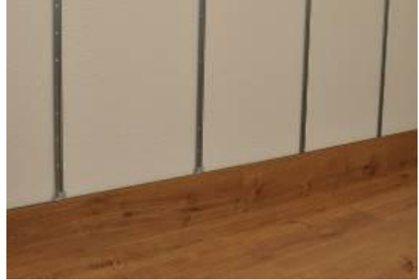
8. Install the first row from left to right and lock the individual boards to the edge joints.
